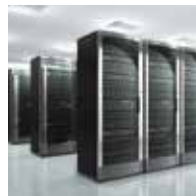
Data Center & Cloud Infrastructure
